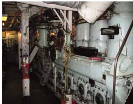
Figure 4. The 1929 Fairbanks Morse engine in the ferry Champlain to be replaced with a new cleaner and more fuel efficient Tier 2-compliant engine (photo by Harold Garabedian).
